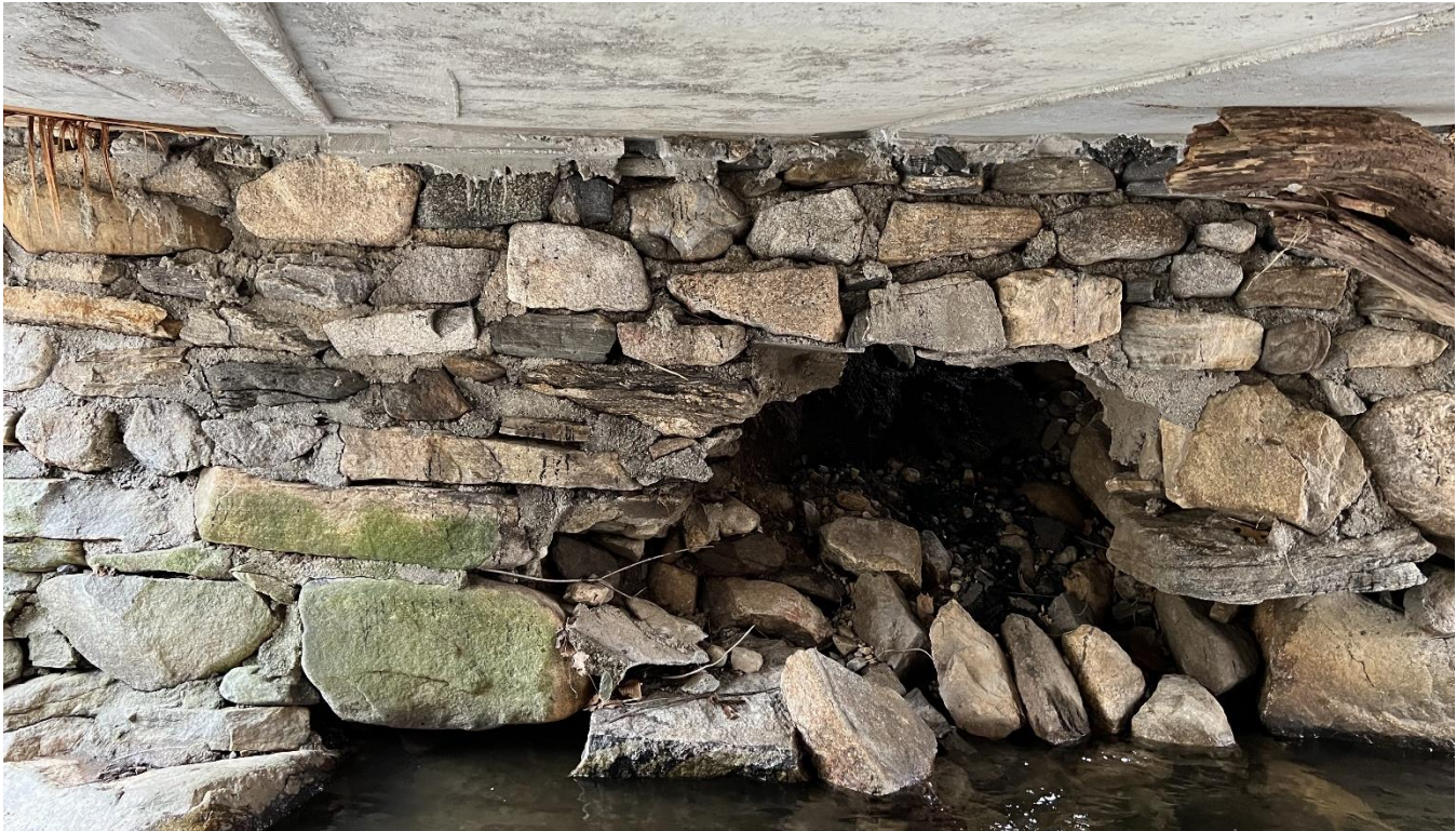
Photo Number: 9 East abutment. Note collapse with daylight visible through southeast wingwall. Photo Taken: 03/14/2025
