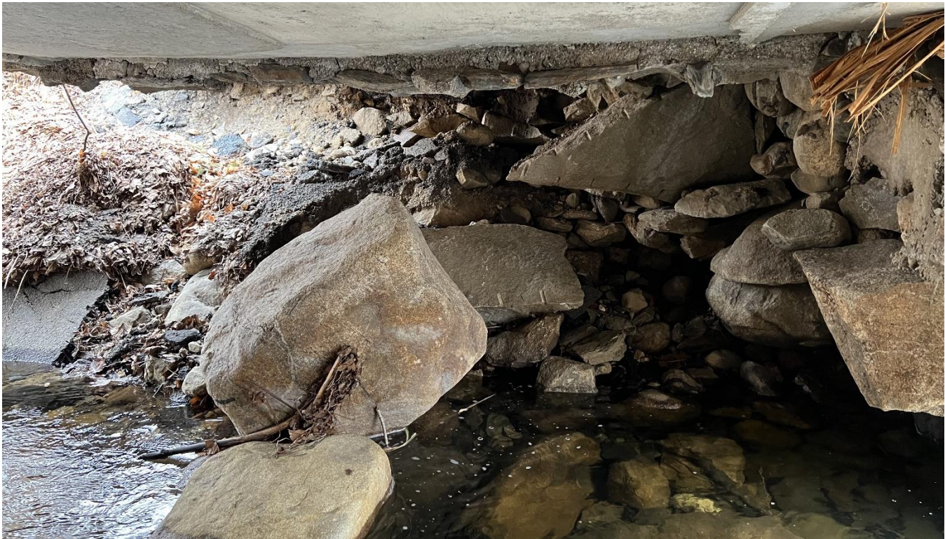
Photo Number: 10 West abutment. Note southern 80% of abutment collapsed/washed downstream. Photo Taken: 03/14/2025
