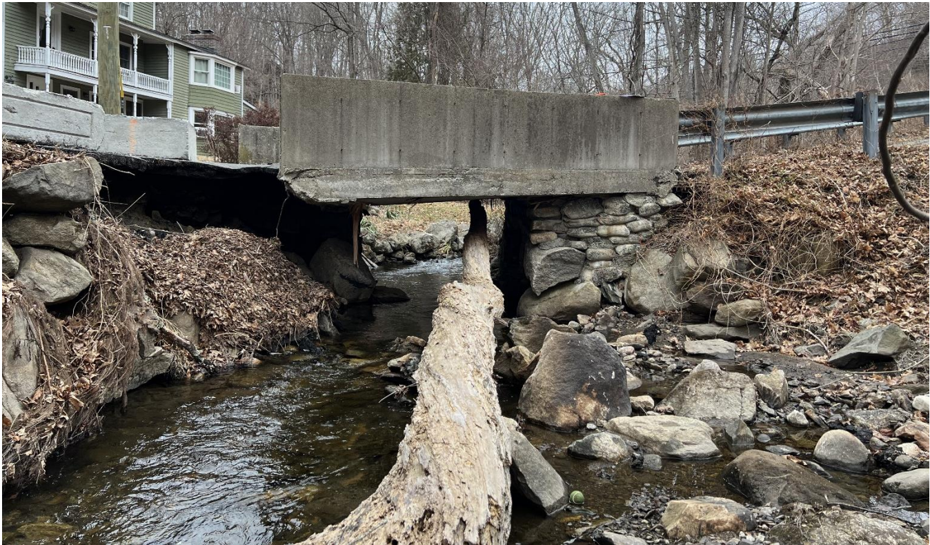
Photo Number: 6 South (downstream) elevation. Note missing abutment, wingwall, and backfill at southwest corner. Photo Taken: 03/14/2025
