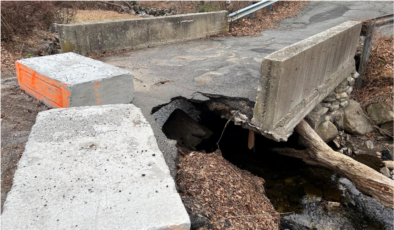
Photo Number: 3 Bridge from west approach. Note collapsed pavement and missing abutment. Photo Taken: 03/14/2024
