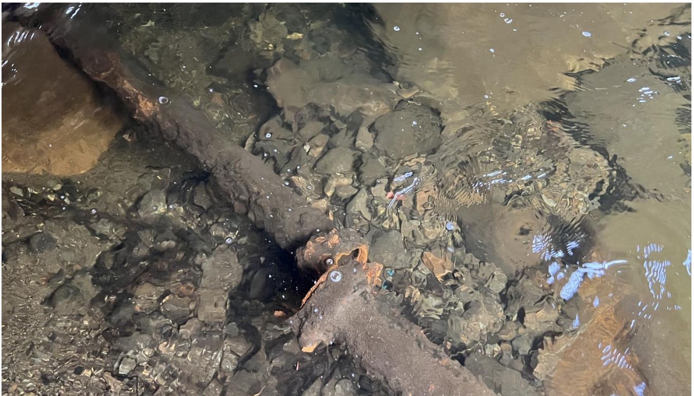
Photo Number: 12 Abandoned utility pipe, with break in pipe Photo Taken: 03/14/2025 clearly visible beneath bridge.
