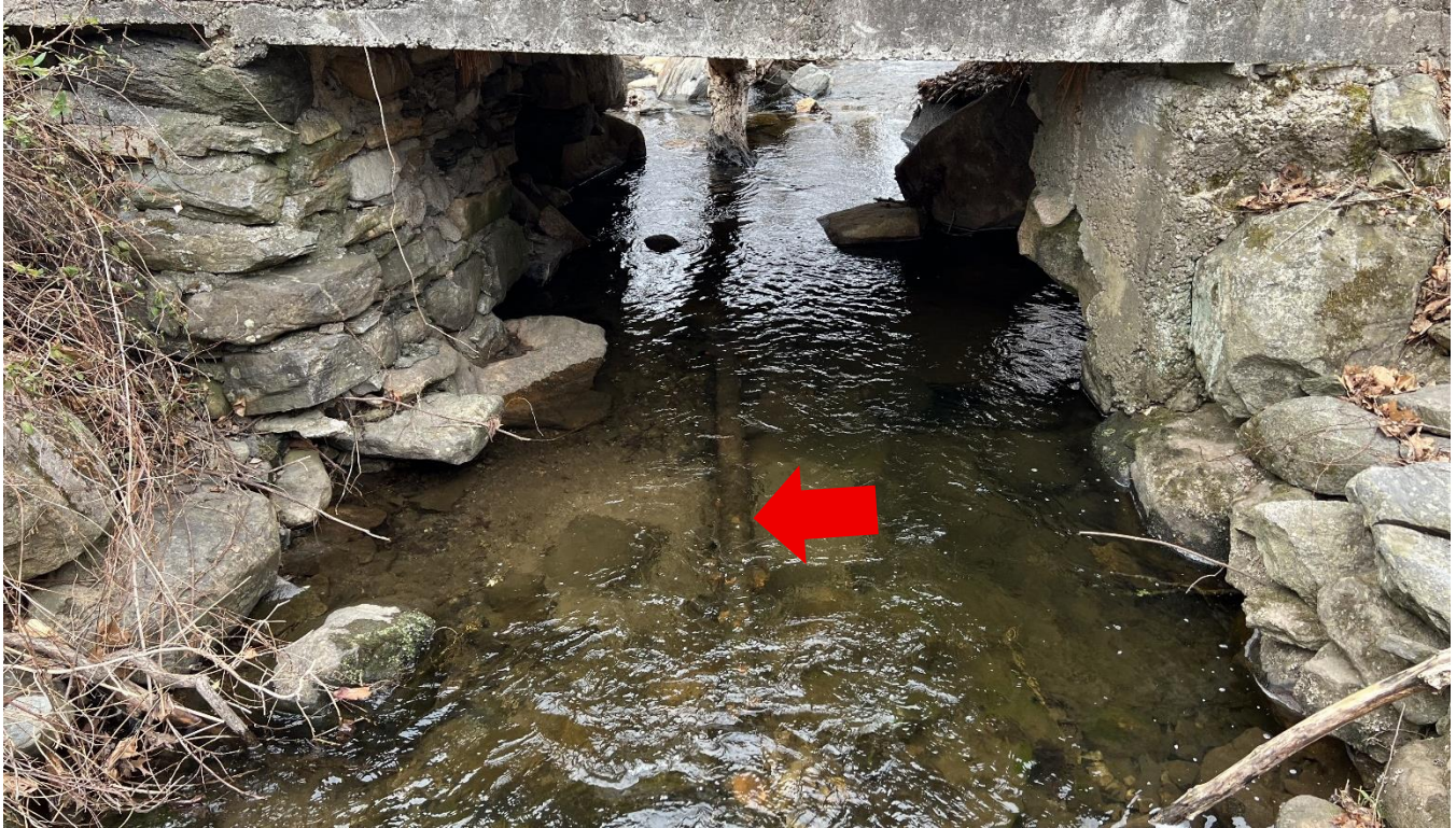
Photo Number: 11 Abandoned utility pipe resting on streambed Photo Taken: 03/14/2025 (looking downstream).
